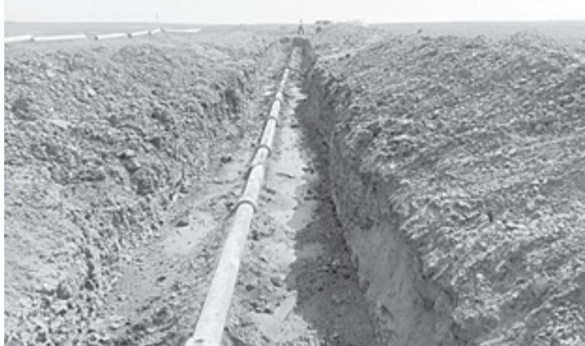
Trench dug by Water Supply workers searching for a broken section of pipeline
