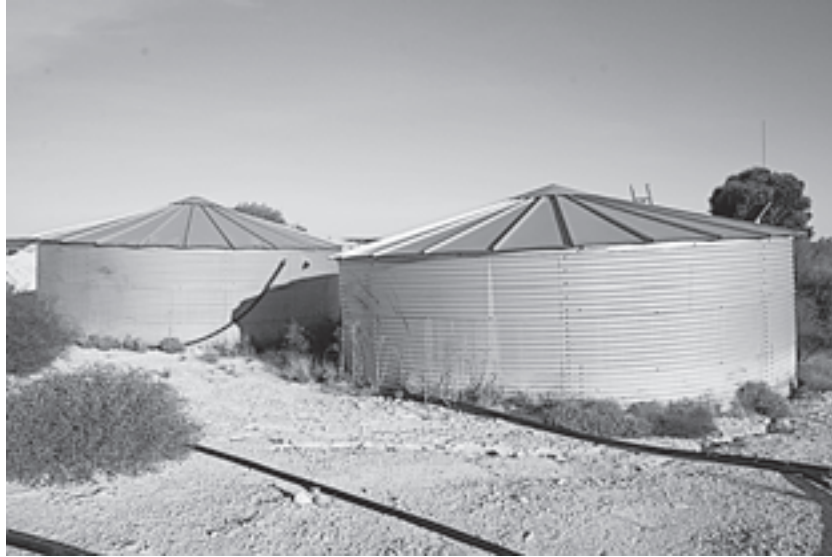
Mintabie water tanks sinking into the ground
